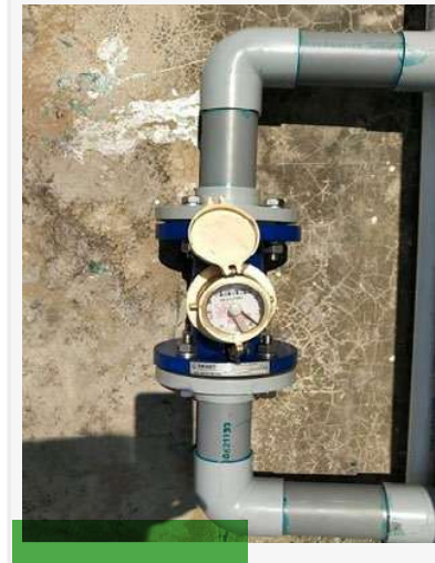
Water flow meters installed in various units for continuous monitoring of Fresh Water and Waste Water
